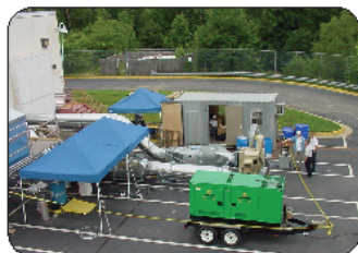
Large scale VHP decontamination system deployed at the U.S. State Department mail processing center in Sterling, Virginia.
